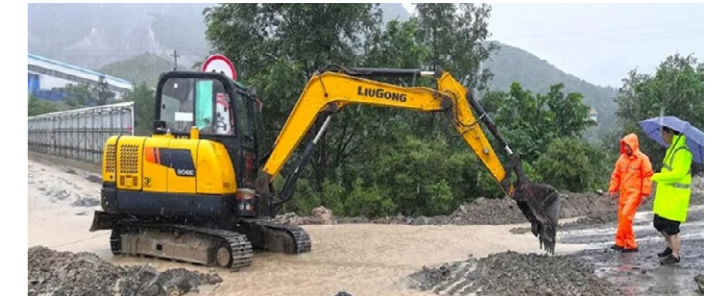
Maintenance personnel are dredging and changing the direction of water flow on the bridge floor
